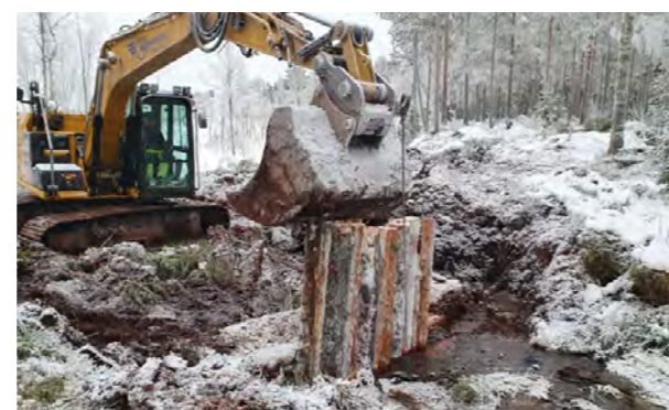
Blocking and filling in a ditch during the wetland restoration at Stormyran in November 2020. Trees from the peatland were cut to reduce evapotranspiration and then used as material to block the ditches. Photo: Tobias Eriksson
