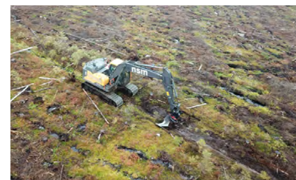
An excavator performing ditch-cleaning. Note that soil mounding had already been performed as a soil preparation method when this photo was taken. Photo Ragna Lestander
