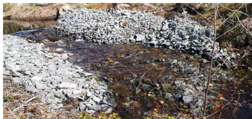
The photo shows a threshold that can be built in ditches with a steeper slope. The water velocity slows down and reduces the risk of erosion. Photo: Mikael Sandberg
